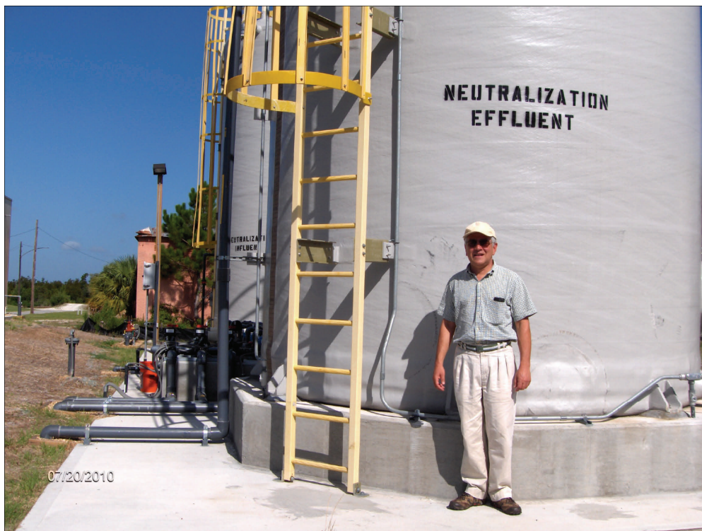
Galo Jackson, EPA Remedial Project Manager for the LCP Chemicals Superfund Site, stands next to one of the tanks installed to treat the Caustic Brine Pool. Due to disappointing treatment results, other technologies are being considered to reduce migration of contaminated groundwater.
